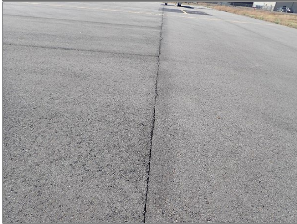
AP-01-11: L&T Cracking
