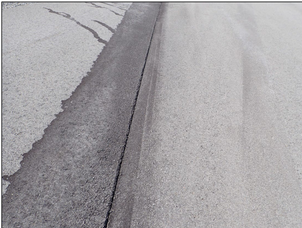
TW-06-03: L&T Cracking
